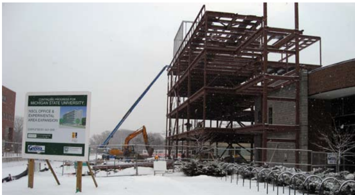
Work to erect the steel superstructure of the office addition started December 15, 2008 and will continue into 2009
